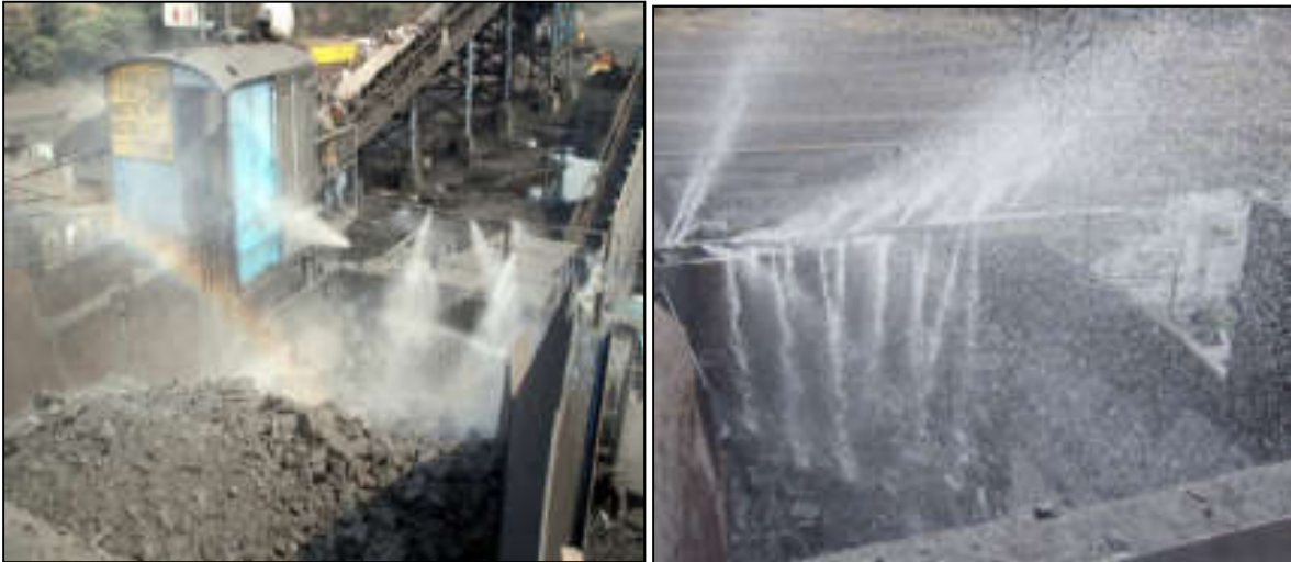
Fig-1: Mist Sprinkler Arrangement at Feeder Breaker
